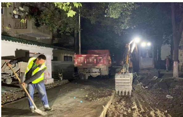
emergency and lighting for small construction operation
